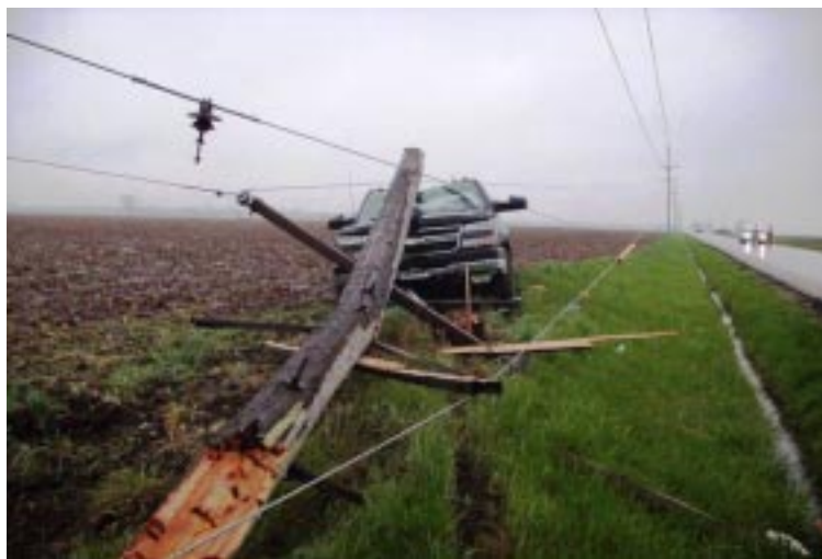
A shattered utility pole remains atop the damaged pickup truck with de-energized lines still attached. (Photo By: Bill Hart/RECC)
